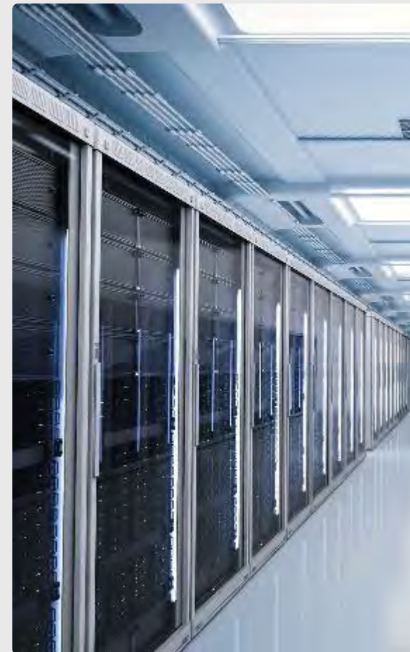
Mission Critical Facilities and Data Centers
