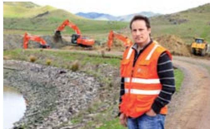
Craig Scott gave his personal reflections on managing the dam emergency at Haldon range Dam. The photo shows equipment excavating the 4m lowering trench on the dam left abutment.
