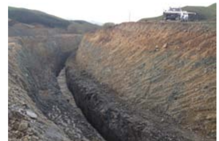
Excavation of the dam left abutment trench to lower the reservoir 4m. Discharge flow visible in the narrow cut at the base of the wide trench.
