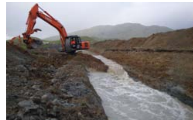
Excavation works in the spillway channel to lower the reservoir 1m. Excavating from the downstream spillway plunge pool back to the reservoir.
