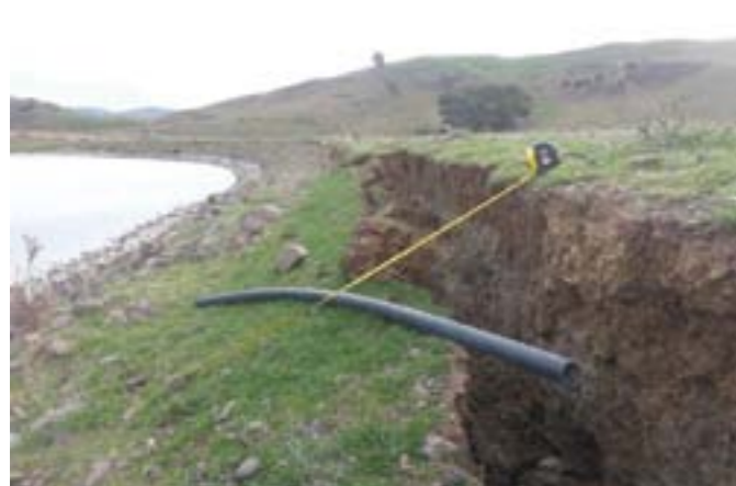
Example dam upstream face slumping crack. This cracking extended the full length of the crest.
