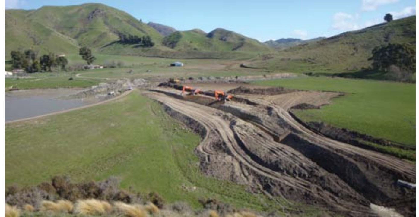
Panorama view to the dam face with the extent of the excavation works to lower the reservoir 4m shown visible on the left abutment.
